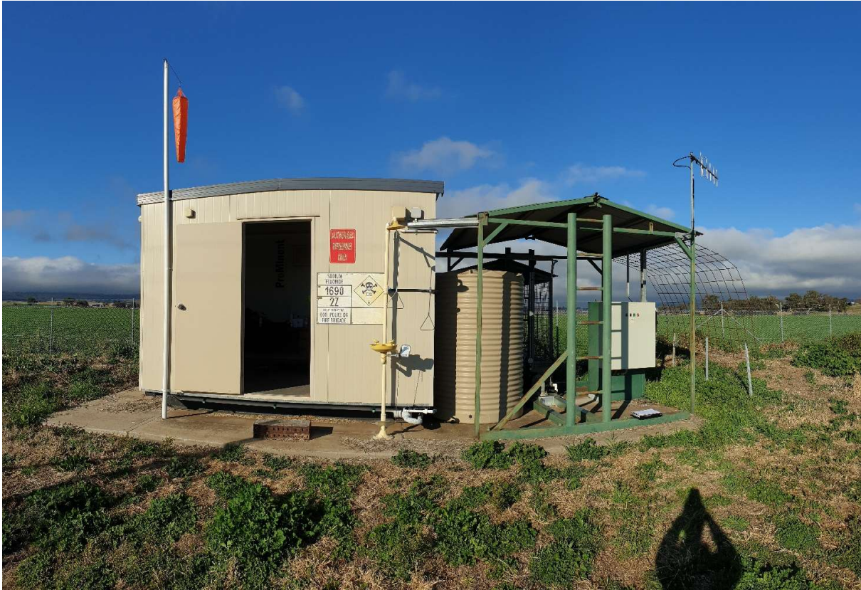
Figure 5-3 Fluoride dosing room at the main bore field
