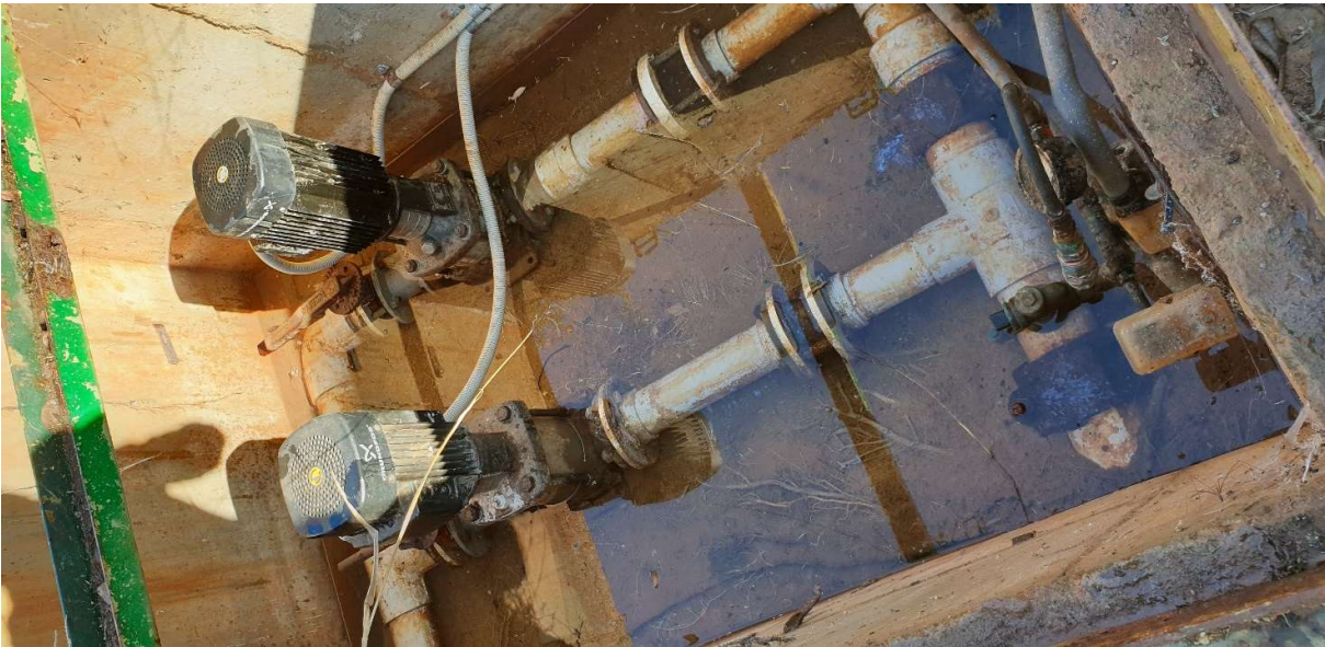
Figure 5-7 Pumping pit for booster pumps near Wentworth Ave reservoir
