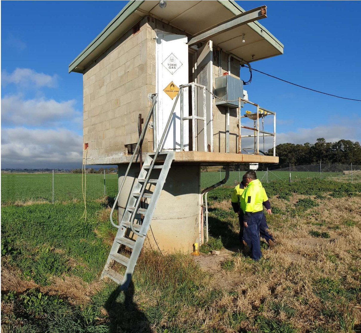
Figure 5-4 Elevated concrete chlorine dosing structure at the main bore field
