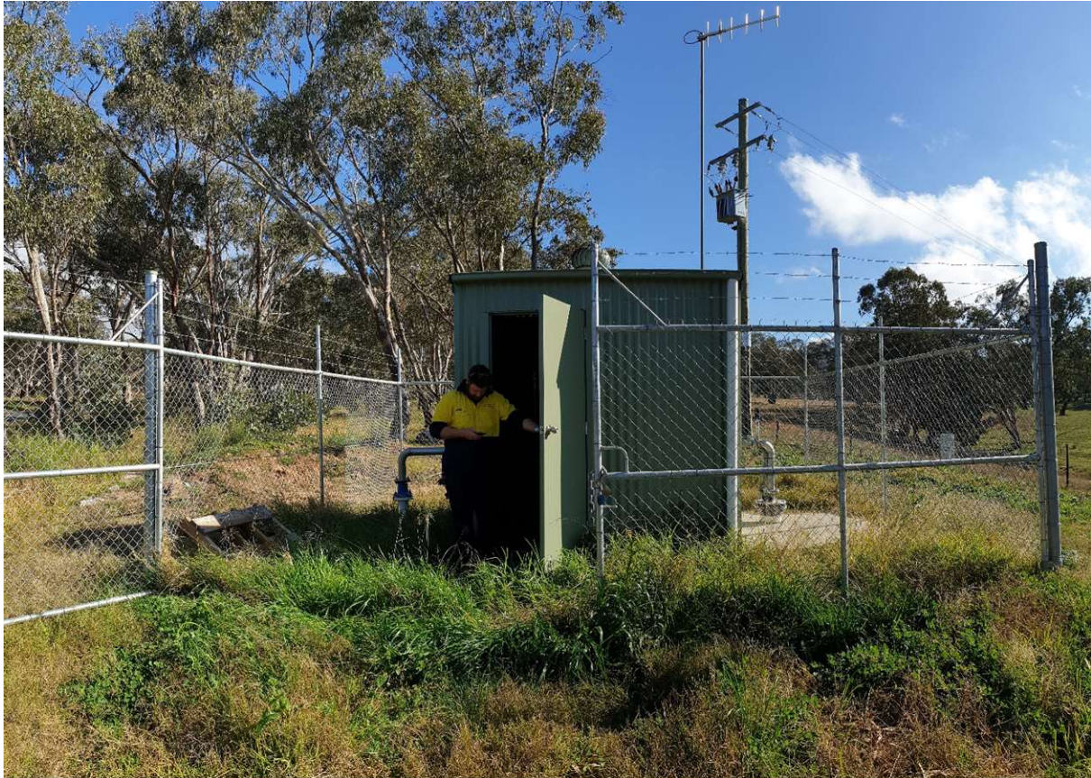
Figure 5-8 Neilrex Rd backup bore site
